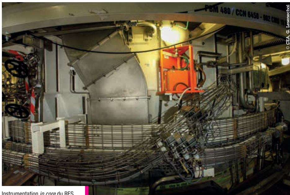
Instrumentation in core du RES.
